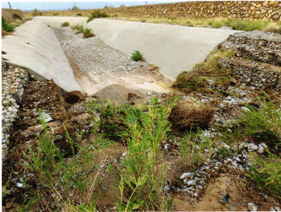
Photograph 10 – 1-2 MID, standing water (8/18/2022).
