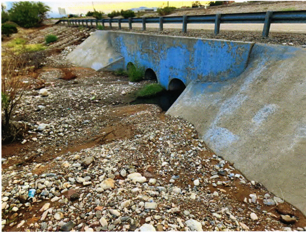
Photograph 3 – 1-6 UP, standing water (8/18/2022).
