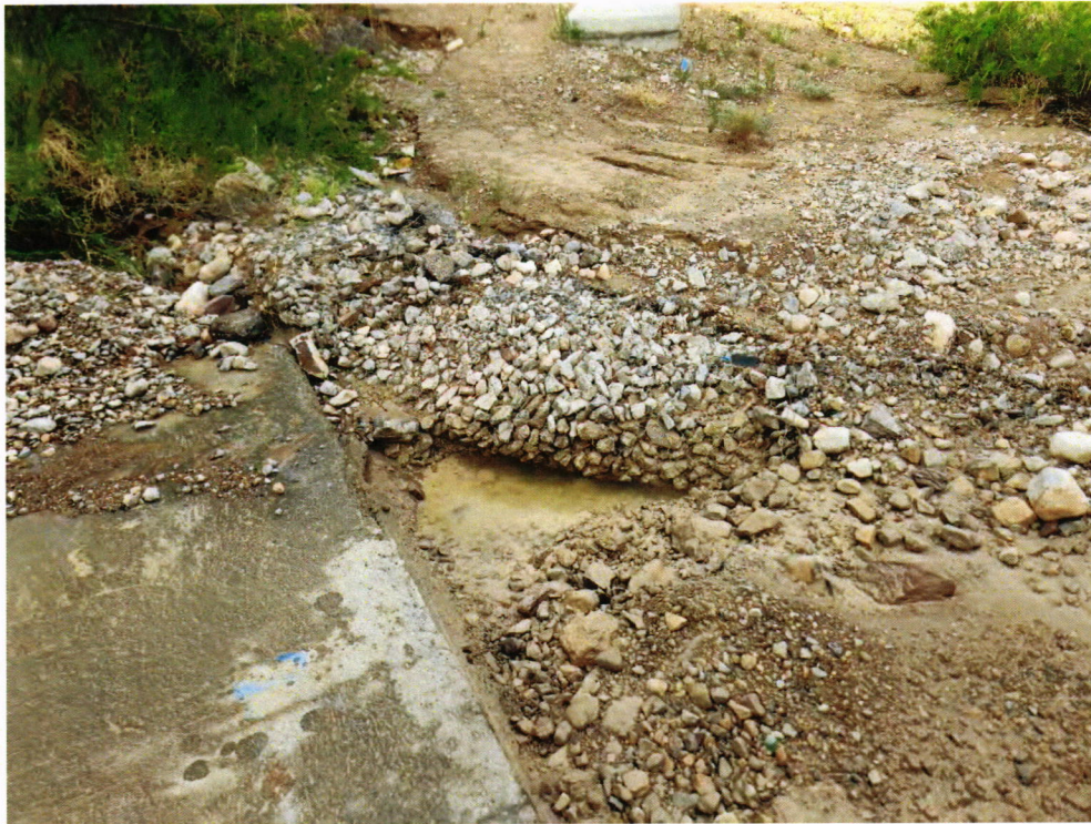
Photograph 8 – 1-1 UP, standing water. (8/18/2022).
