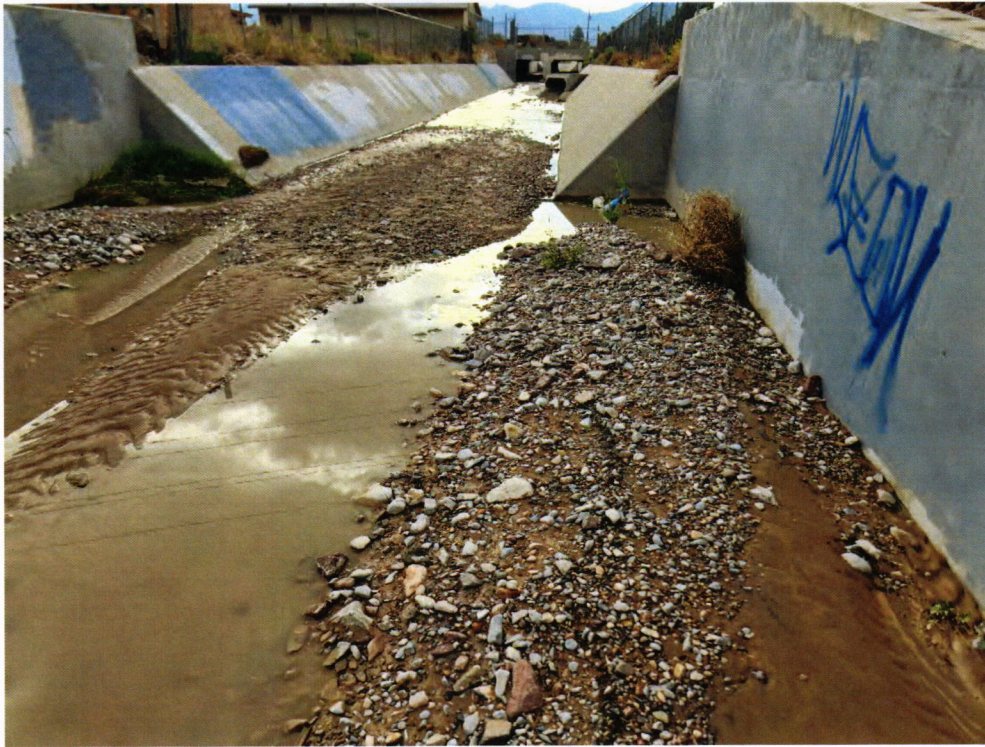
Photograph 9 – 1-1 MID, standing water (8/18/2022).
